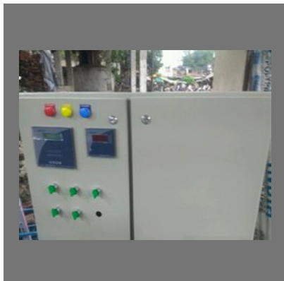
Three-Phase Control Panel
