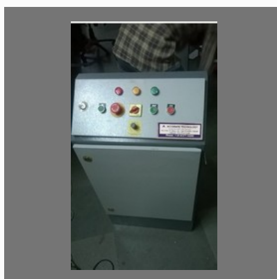
Electric Control Panel
