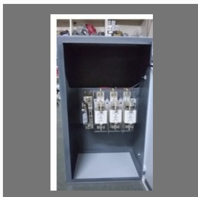
Electric Control Panel
