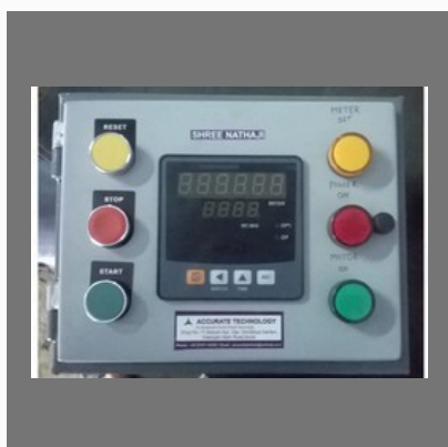
Electric Control Panel
