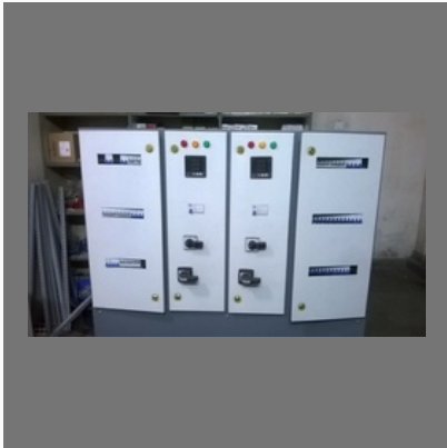
PDB Control Panel
