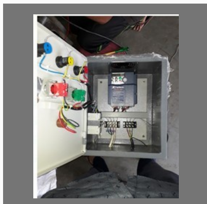
Single Phase Control Panel
