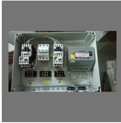
Aerators Control Panel
