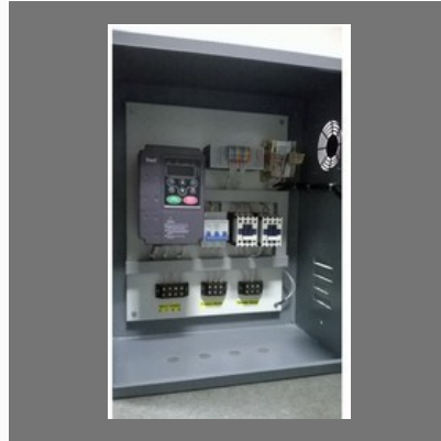
Electric Control Panel
