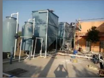
Commercial Sewage Treatment Plant
