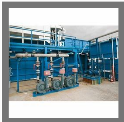
Effluent Treatment Plant
