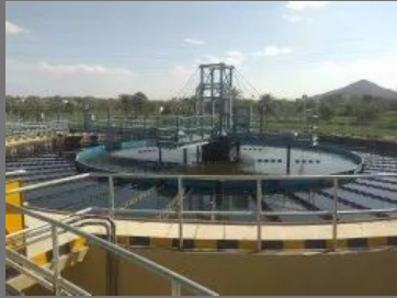
Effluent Treatment Plants
