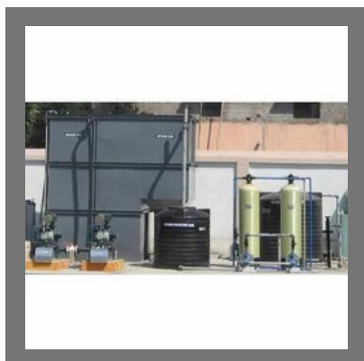
Sewage Treatment Plant
