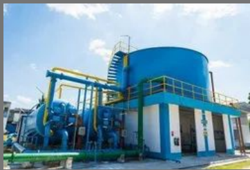
Industrial Sewage Treatment Plant
