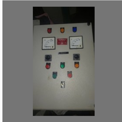
Motor Starter Panel
