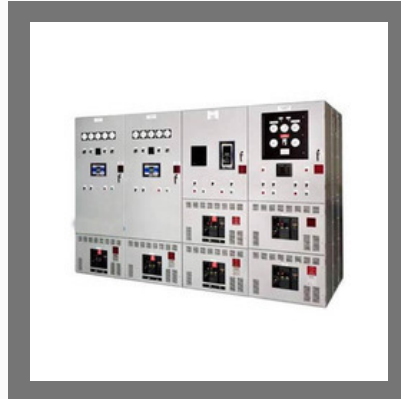
LT Distribution Panel
