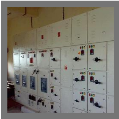
LT Control Panel
