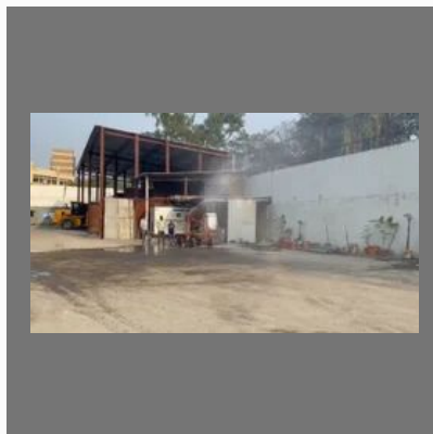
dust suppression system
