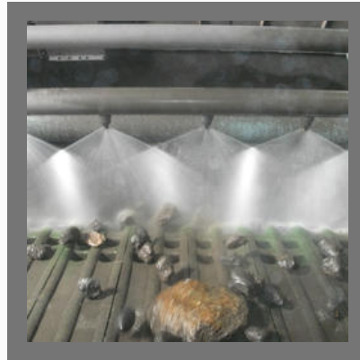
Dust suppression system
