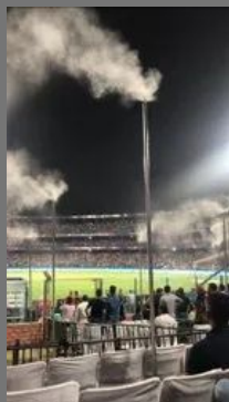
High Pressure Misting System
