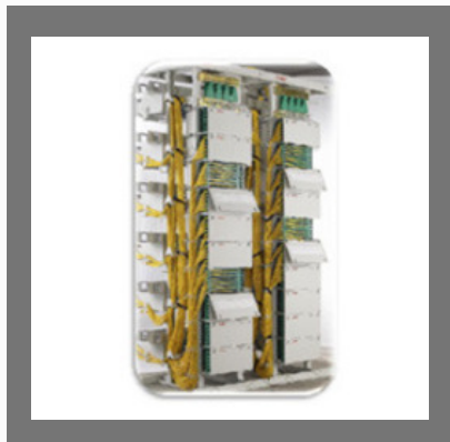
Optical Main Distribution Frame
