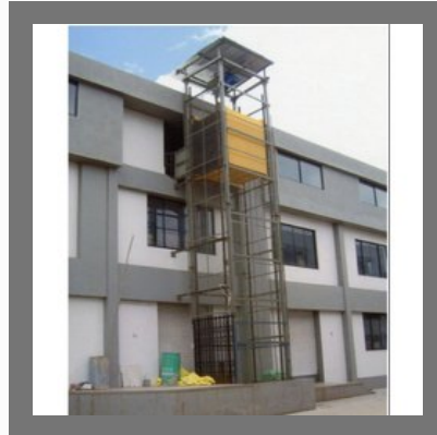
Commercial Goods Lift
