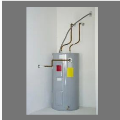
Electric Water Heater
