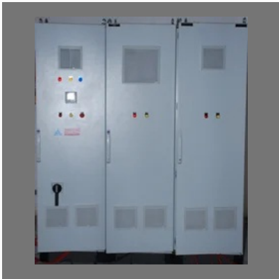
Drive & Process Automation
