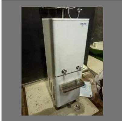
Drinking Water Coolers
