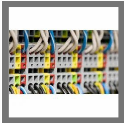
Internal Electrification Services
