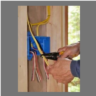
Electrical Wiring Services
