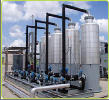
Biogas Purification Plant
