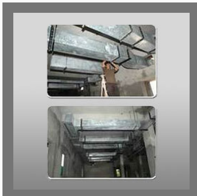
Industrial HVAC Ducts
