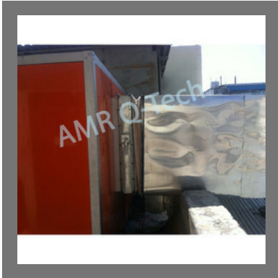
Air Handling Unit
