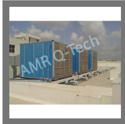
Centralized Air Cooling System
