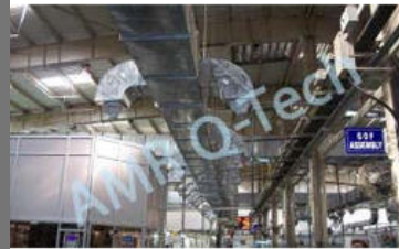
Air Distribution System
