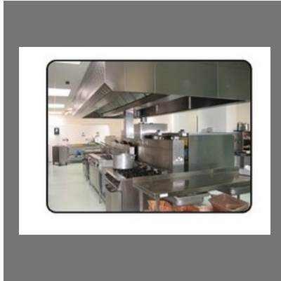
Kitchen Hoods for Exhaust
