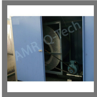
Air Cooling System
