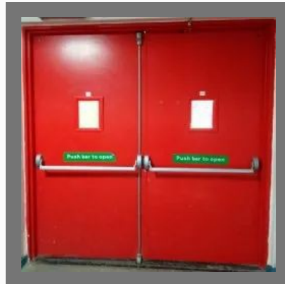
Emergency Exit Fire Door
