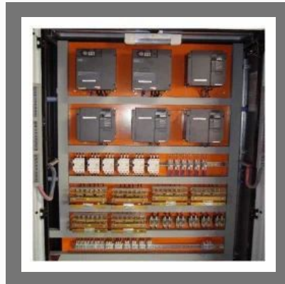
Vfd Electrical Panel
