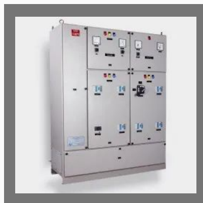
Electric Control Panel
