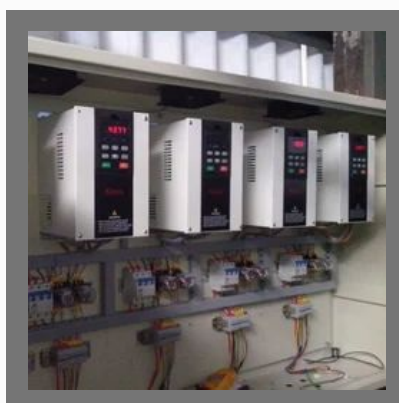
VFD Control Panels
