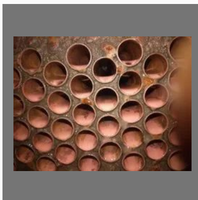
Descaling Of Condenser
