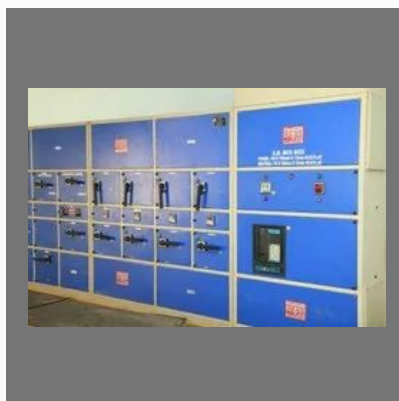
Mcc Electrical Control Panel Services
