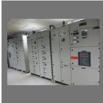
Low Voltage Control Panel & Services
