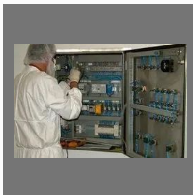
Electrical Control Panel Service
