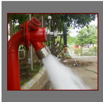
Fire Hydrant Valve
