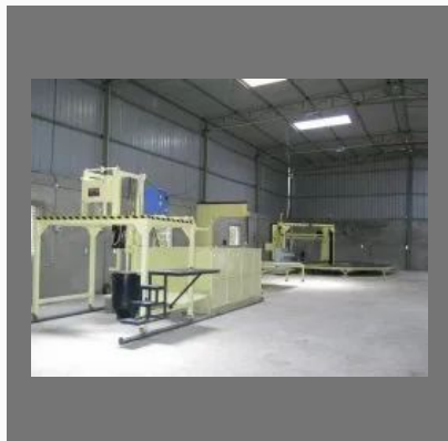
Rebonded Foam Plant
