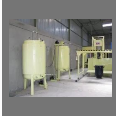
Rebonded Foam Plant
