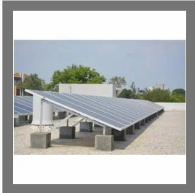
Company Solar Rooftop Plant
