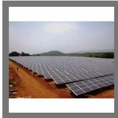
Solar Power Plant
