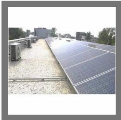
20K WP Solar Rooftop Plant
