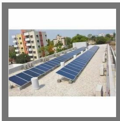
Solar Rooftop Plant
