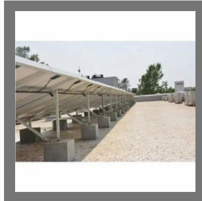
Heavy Duty Solar Rooftop Plant
