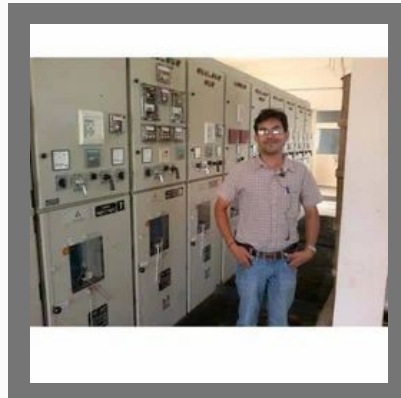
DG Set Auto Control Panel
