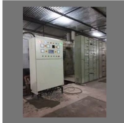
AMF Control Panel
