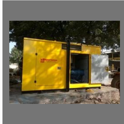
Acoustic Enclosure DG Set
