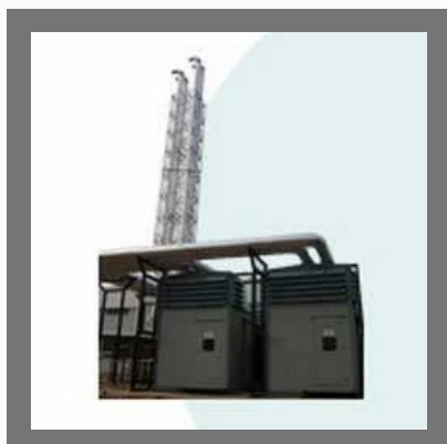
DG Sets Installation Service
