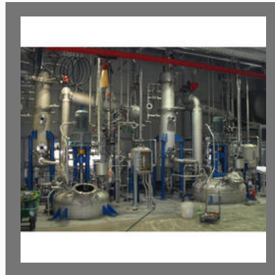
Polyester Resin Plant
