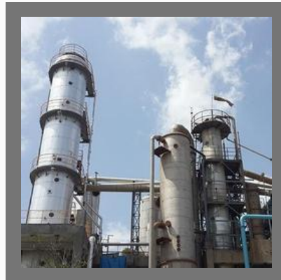
Phenol Formaldehyde Resin Plant
