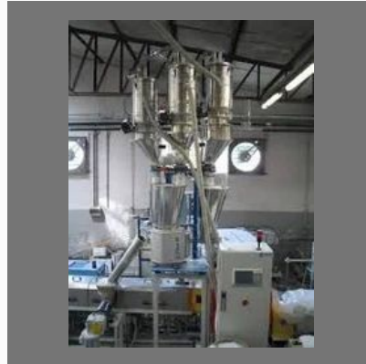
Pneumatic Conveying System
