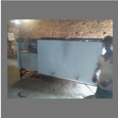
Water Chilling Plant
