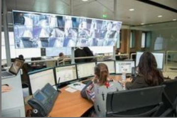
Surveillance CCTV System Services
