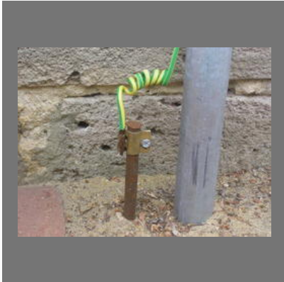
Electrode Earthing System
