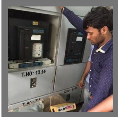
Relays Testing Services
