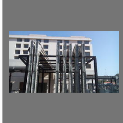
Electrical Bus Duct
