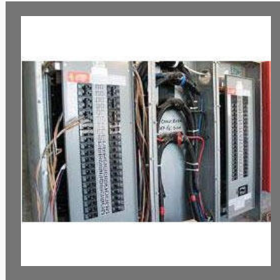
Control Panel Repairing Services
