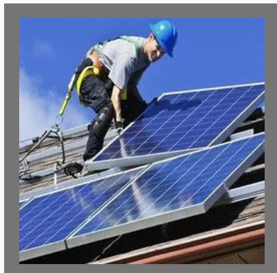
Power Panel Installation Service
