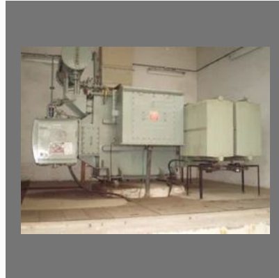
Indoor Type Substation
