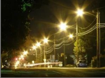
Operation And Maintenance Of Street Lights
