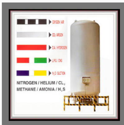
Liquid Oxygen Tank
