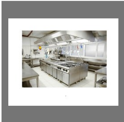
Restaurant Kitchen Equipment
