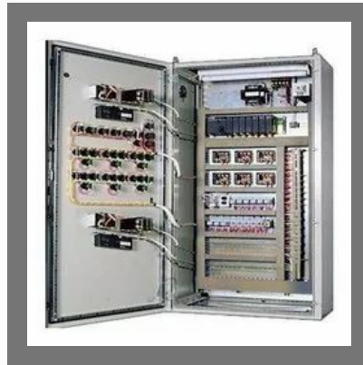
Electrical Control Panel
