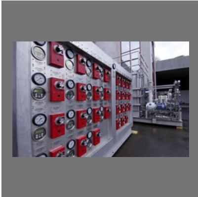
Pressure & Flow Control Panel
