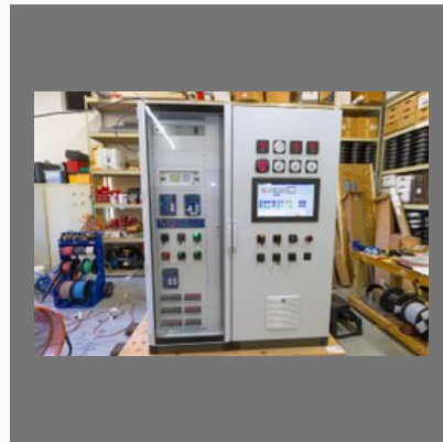
PLC SCADA Automation Control Panel
