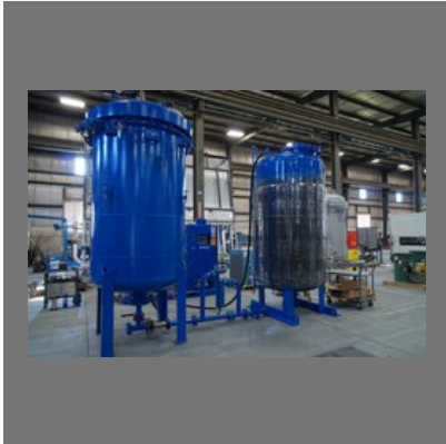
VPI And ED Coating Plant Automation Control Panel
