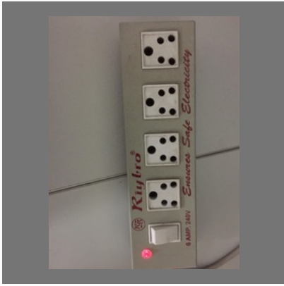
Electrical Switch Board
