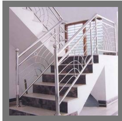
Stainless Steel Hand Railing
