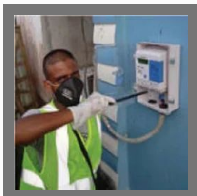
Smart Meter Installation
