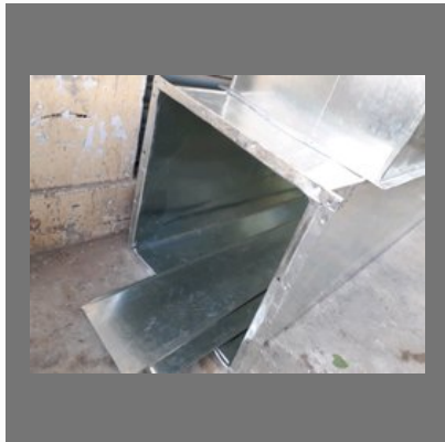
Smoke Exhaust Systems
