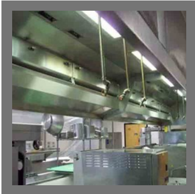
Kitchen Exhaust Hood
