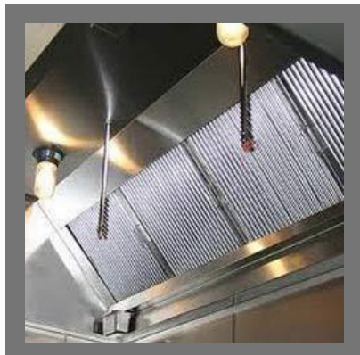
Kitchen Exhaust System
