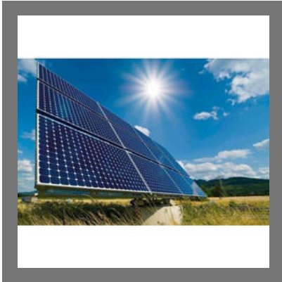
Solar Power System
