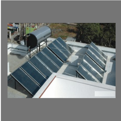
Industrial Solar Water Heater
