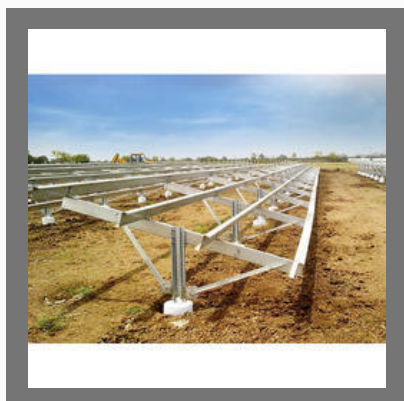
Solar Panel Structure
