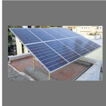
Rooftop Solar System
