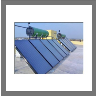
Solar Water Heater
