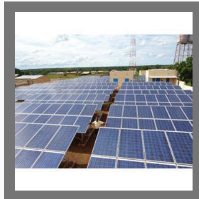
Industrial Solar Panel
