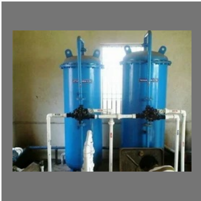
RO Treatment Plant
