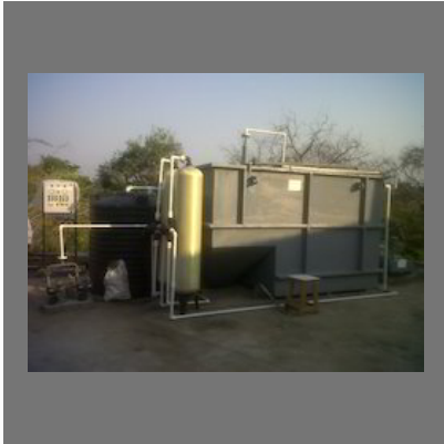
Sewage Treatment Equipment
