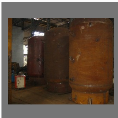
Air Receiver Tank
