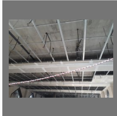
Gypsum Partition Services And Installation Of Gypsum Ceiling And Installation Of Armstrong
