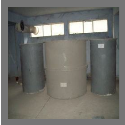
FRP Dosing Tank
