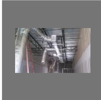
Air Conditioner Ducting
