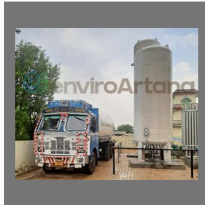
Cryogenic Liquid Oxygen Plant
