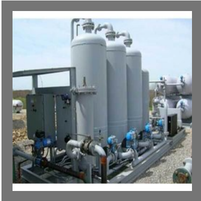
Biogas Purification Plant
