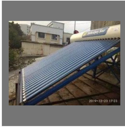
Solar Water Heater ETC
