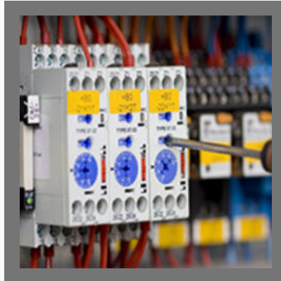
Electrical Solutions Service
