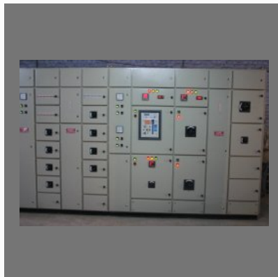
LT Control Panel
