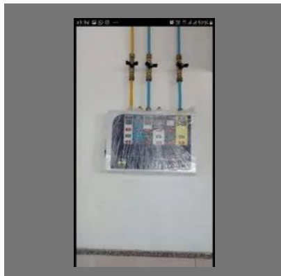
Oxygen Gas Alarm System
