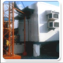
Radio Power(Bts) Maintenance System
