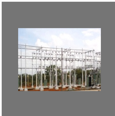
Sub Station Feeder Distribution Systems
