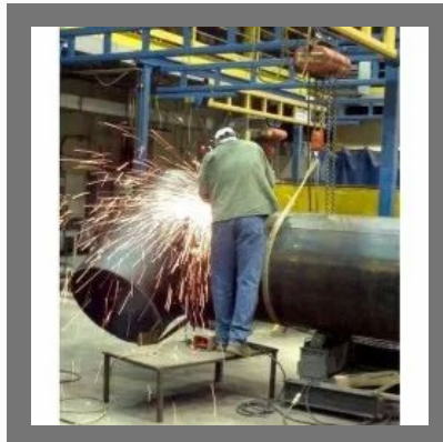
Pipe Fabrication Service
