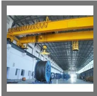
EOT Crane Service
